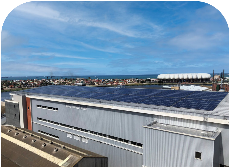
SOLAR PANELS INSTALLED AT ASPEN FLAGSHIP SITE IN GQEBERHA, SOUTH AFRICA, WHICH PROVIDES ACCESS TO QUALITY, LIFE SAVING MEDICINES TO PATIENTS IN AFRICA AND THE WORLD
