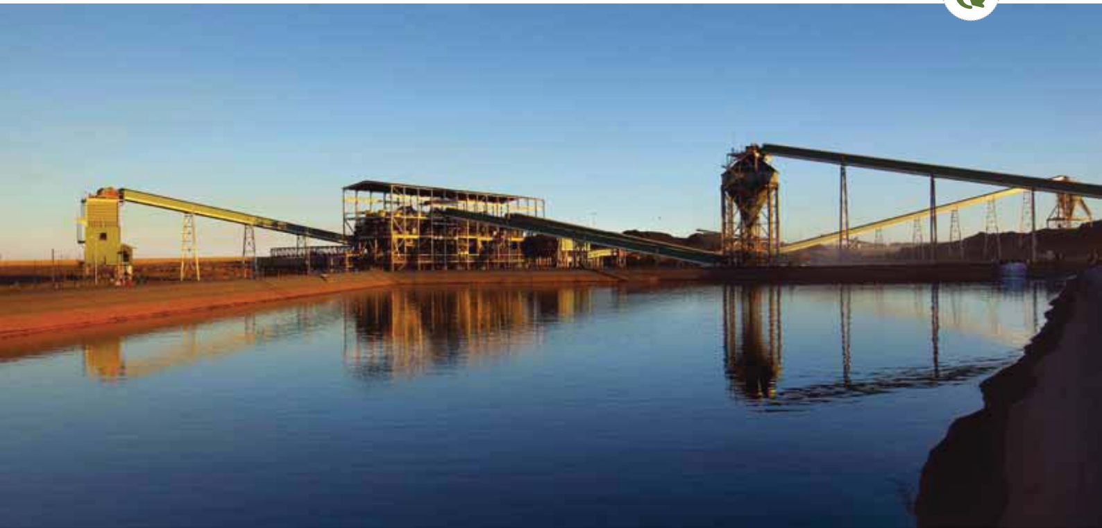
Goedgevonden Mine Coal Handling Processing Plant (CHPP)
