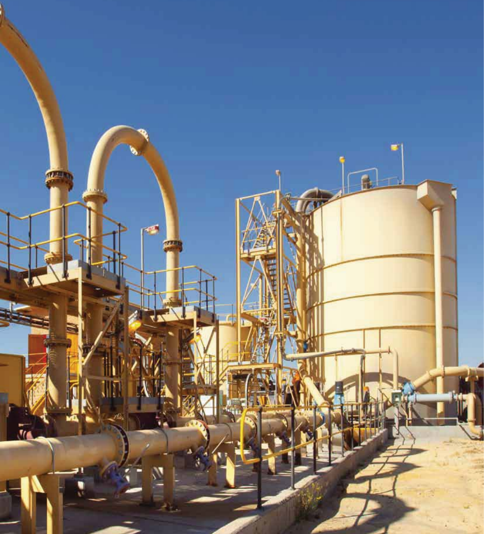
Nkomati Nickel Mine choke station at Onverwacht Tailings Dam
