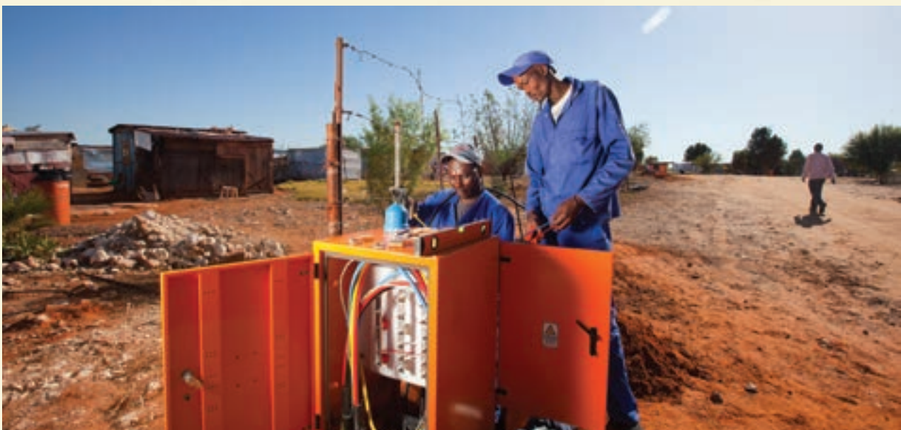
Khumani: Investment in bulk electricity supply and household connections at Mapoteng township
