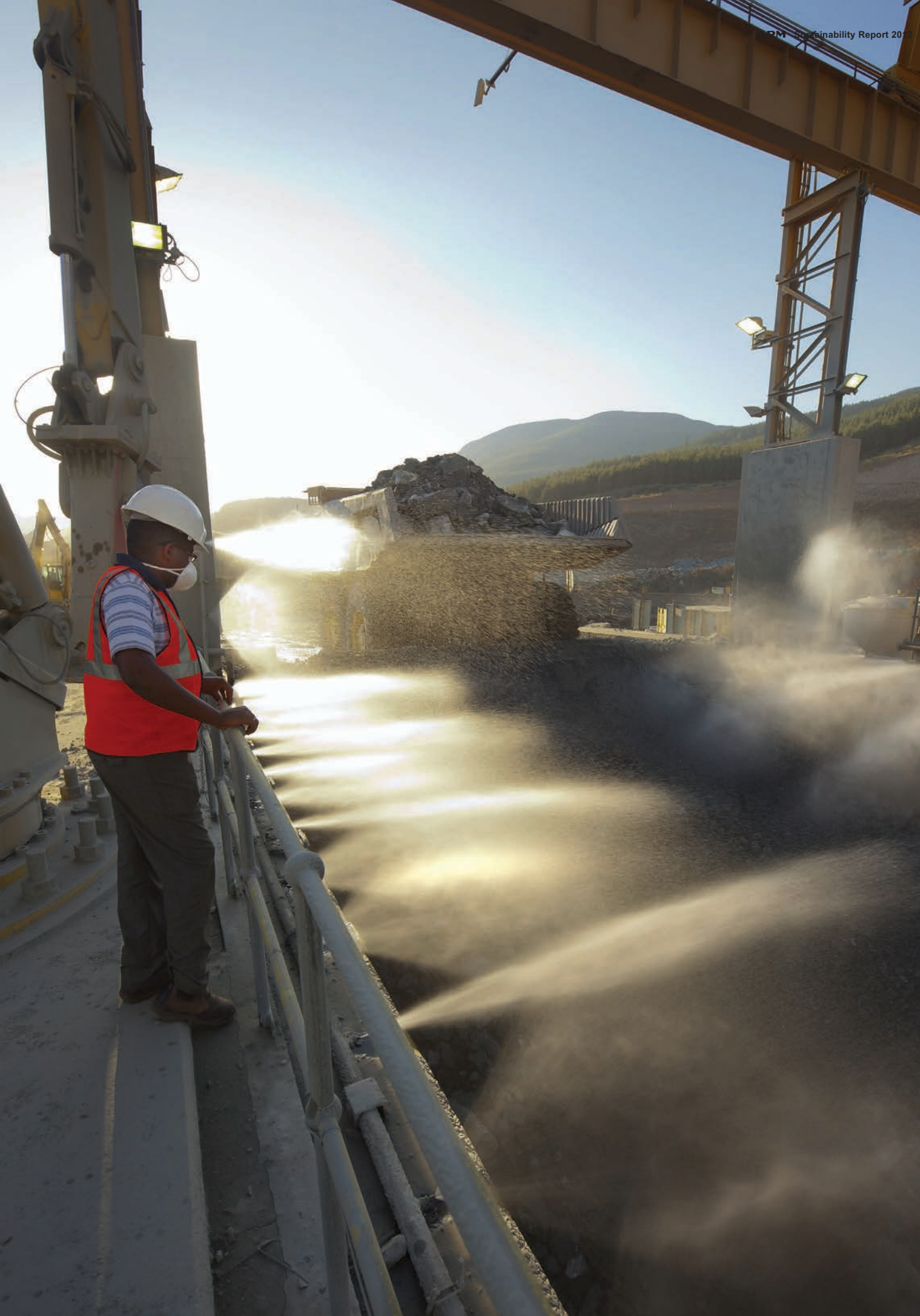
Dust suppression system at crusher, Nkomati Mine
