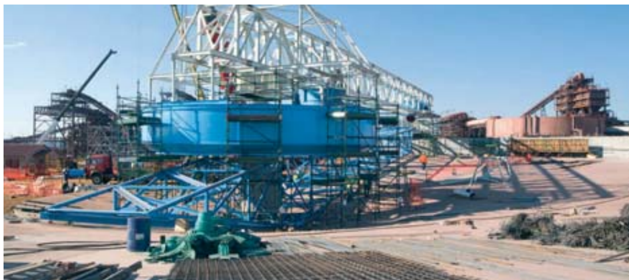
The new thickener at the expansion of Khumani to 16 mtpa
