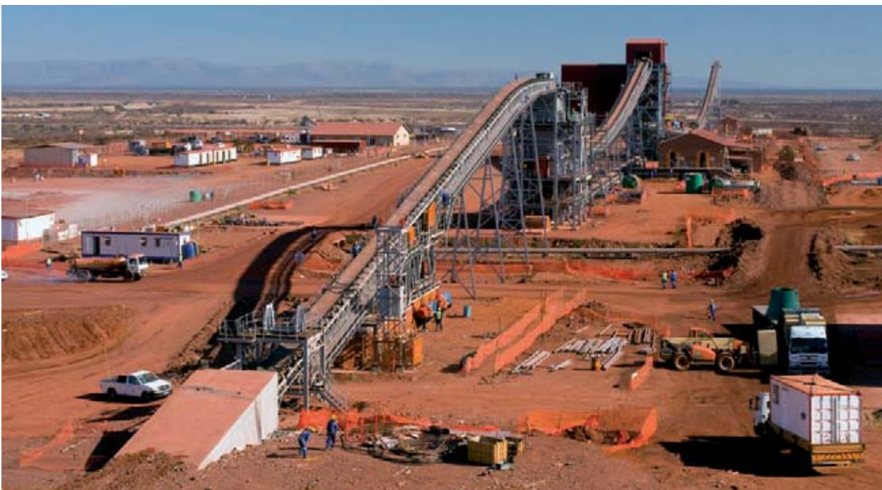
The King Primary and secondary crusher installation under construction at Khumani Mine
