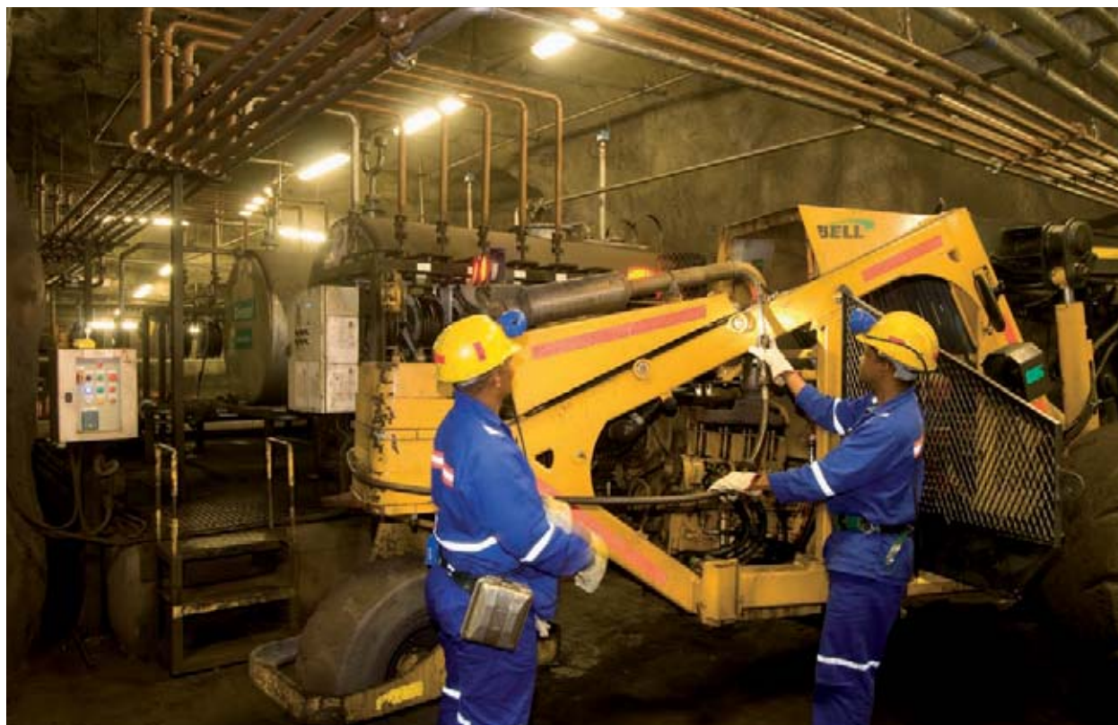
Underground refueling facility at Nchwaning 3 Shaft
