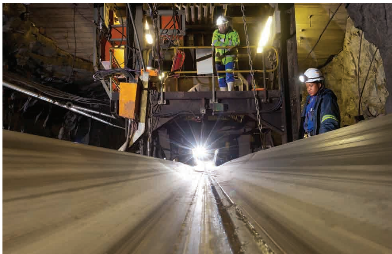
Main portal underground ore pass to conveyor station, Two Rivers Platinum Mine
