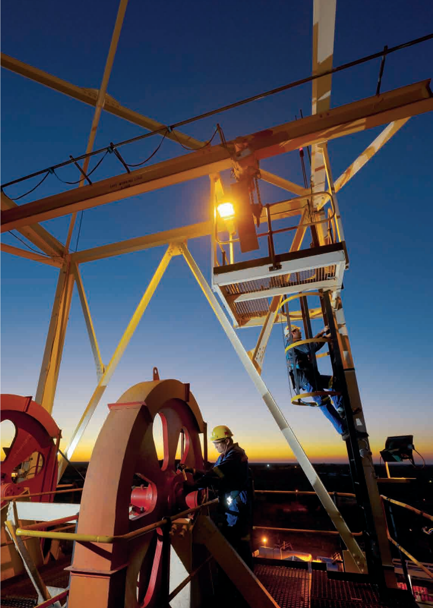
Nchwaning 3 sheaf wheel maintenance
