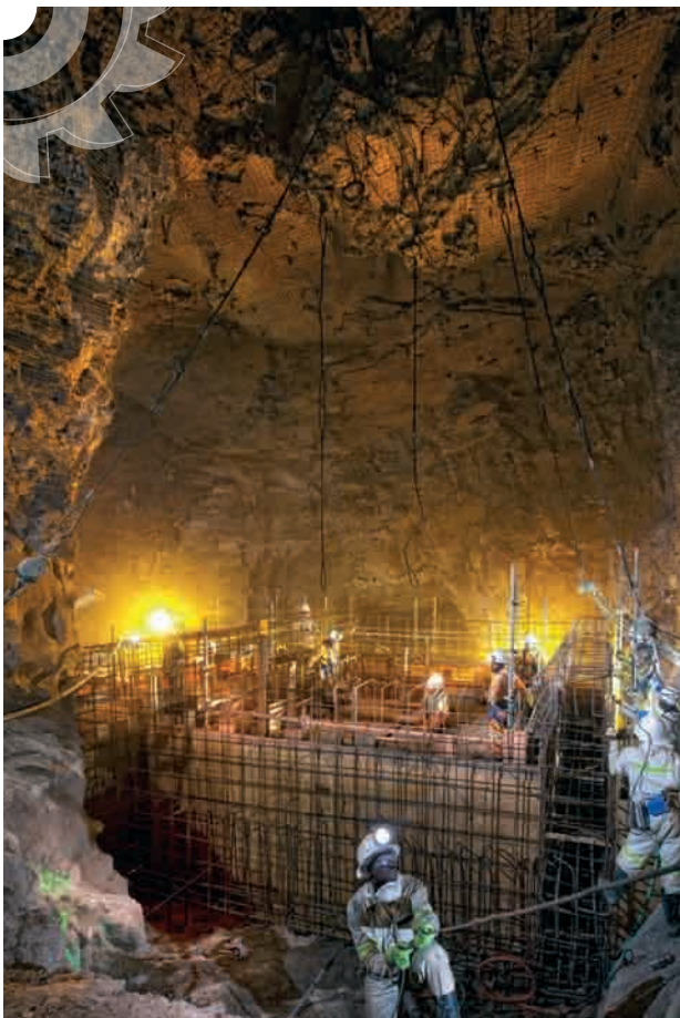
Underground rock transfer system at Lubambe Copper Mine
