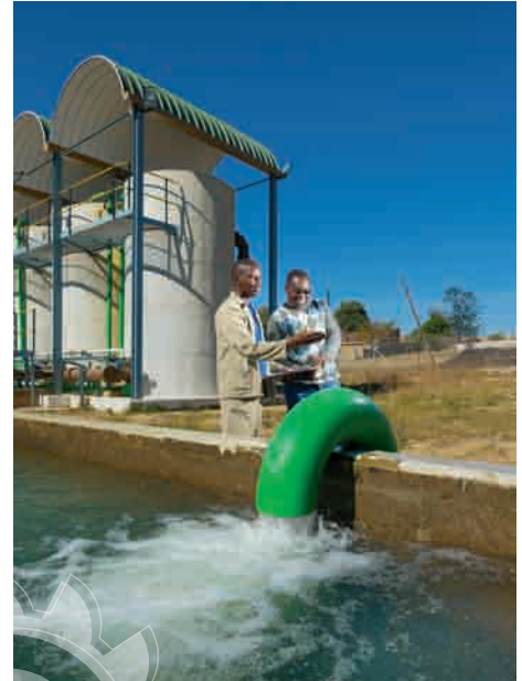
Badplaas water treatment plant upgrade, Nkomati Nickel Mine
