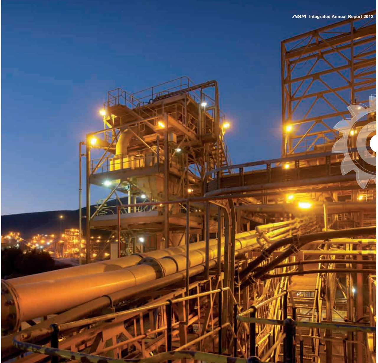
Nkomati Nickel Mine MMZ concentrator plant
