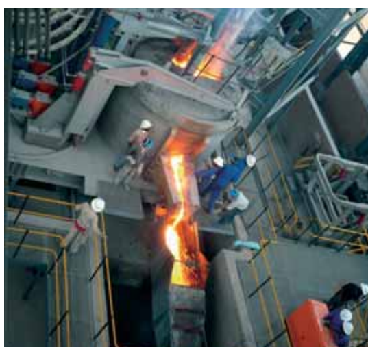
MVA AC ARC Furnace, DRC
