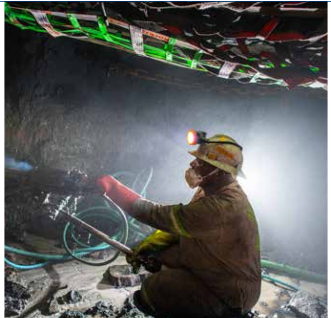
Rock drill operator drilling the face under the protective cover of heavy-duty netting
