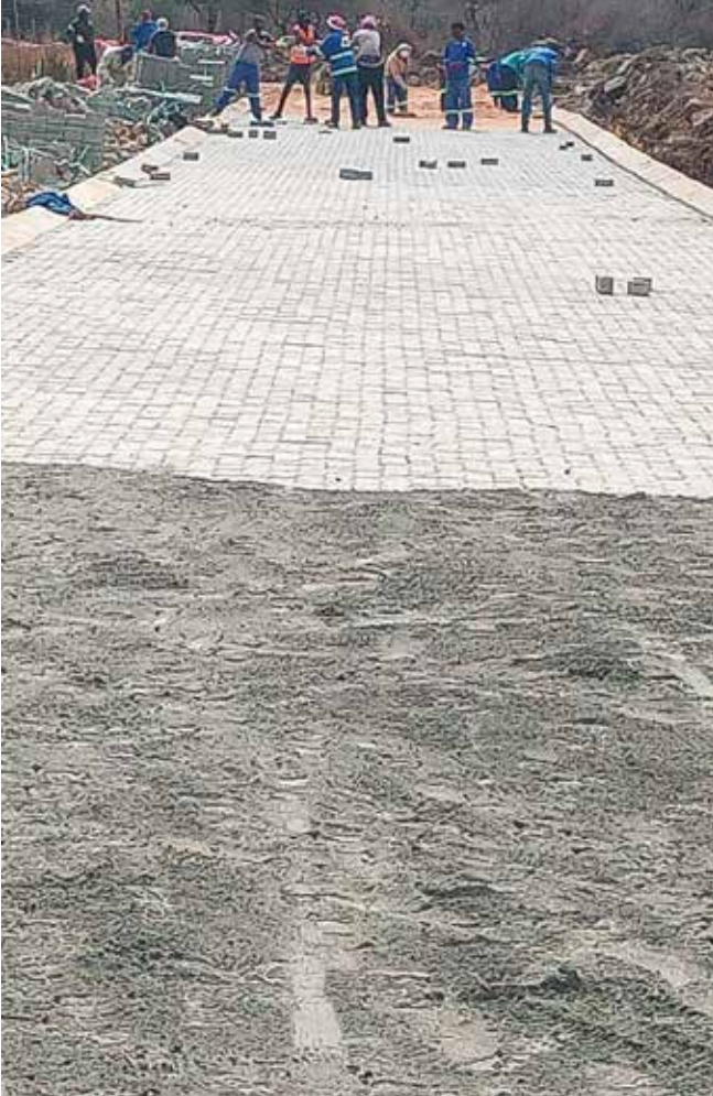
Waste rock from Impala Rustenburg was used in the construction of this road leading to Kutlwanong School for the Deaf
