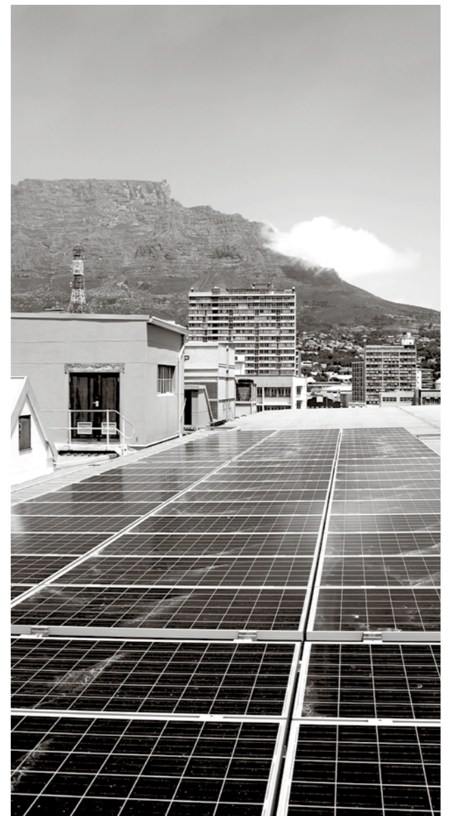
Solar installation at Woolworths head office
